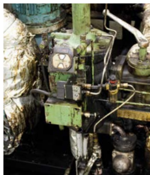
Automatic fuel oil filters.
