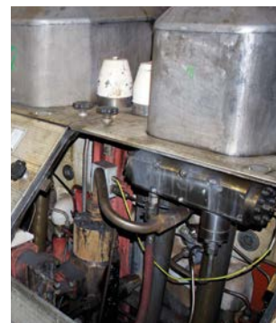
Fuel injection pumps.
